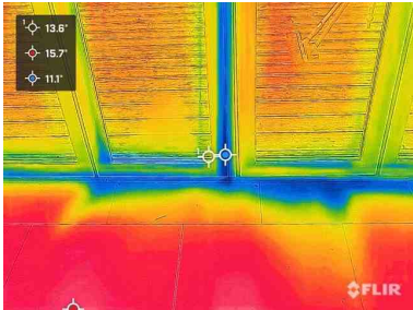
infrared thermography shows draft at failed door seals as a feathering pattern
